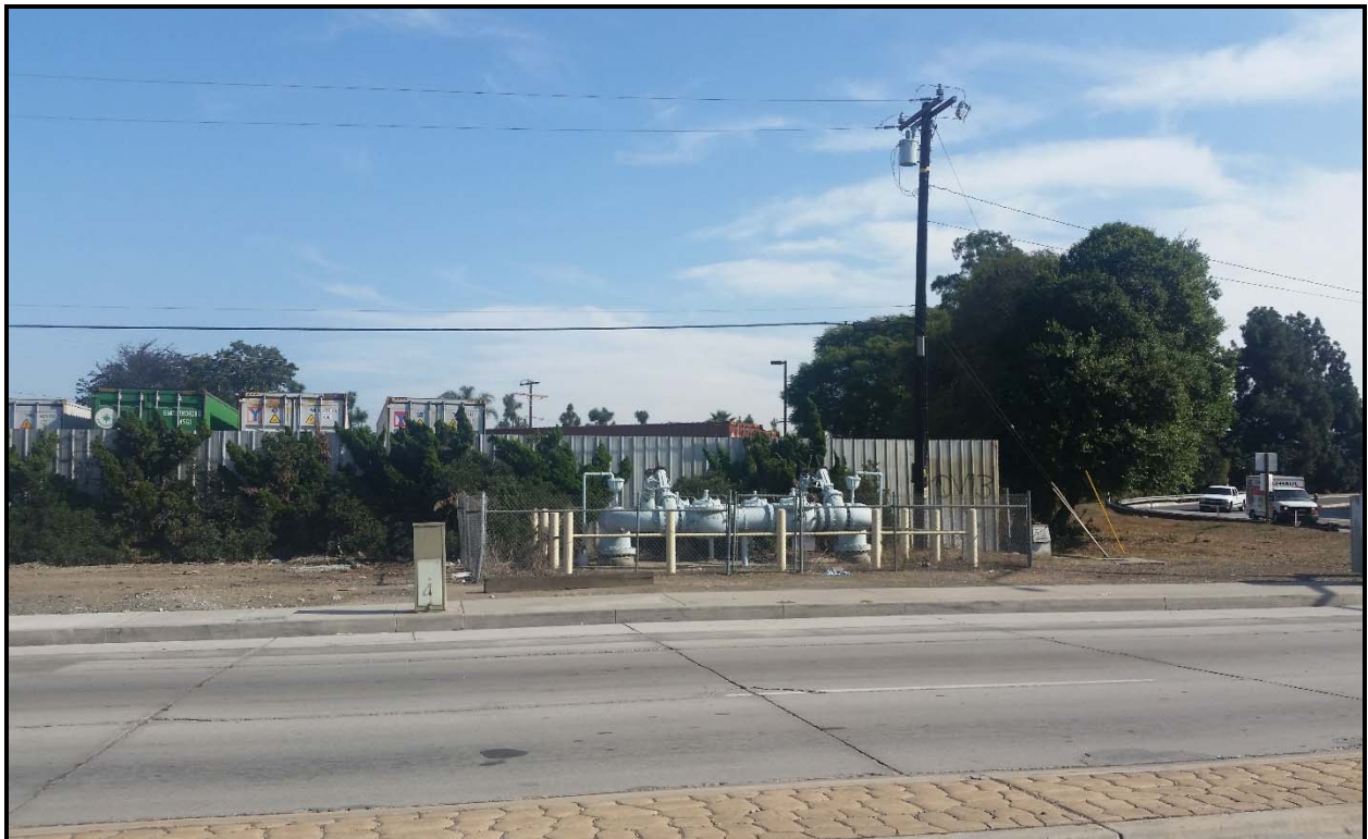
Photo 6. Valve site(?) on Alameda Street. Segment: 3
