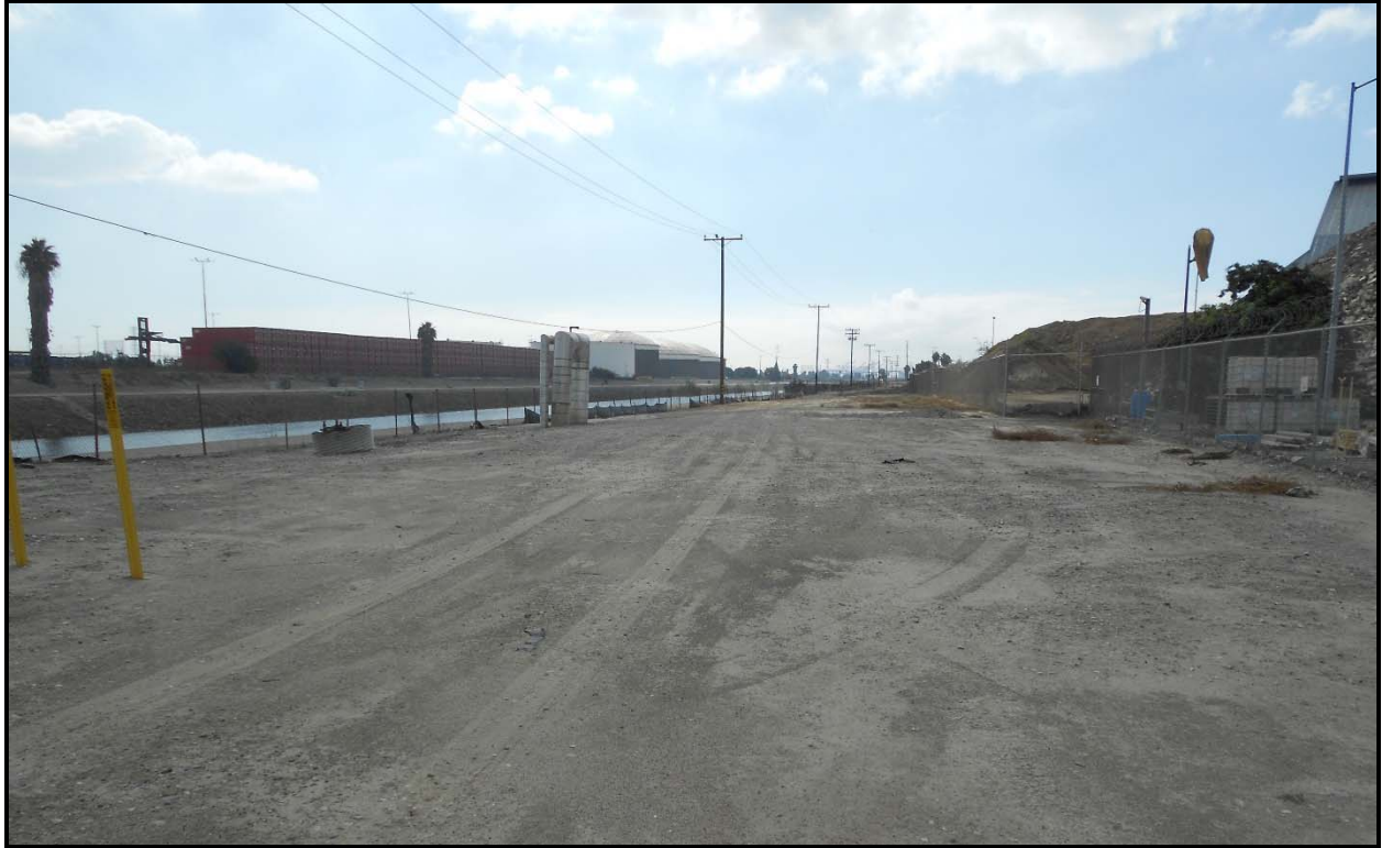
Photo 1. Construction area for one half mile of new pipe at Carson Facility. Segment: 1
