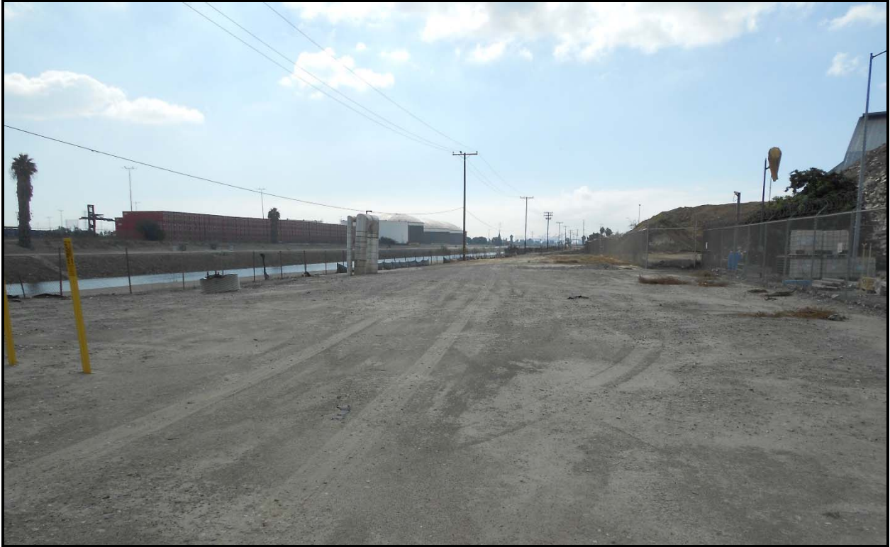
Photo 1. Construction area for one half mile of new pipe at Carson Facility. Segment: 1
