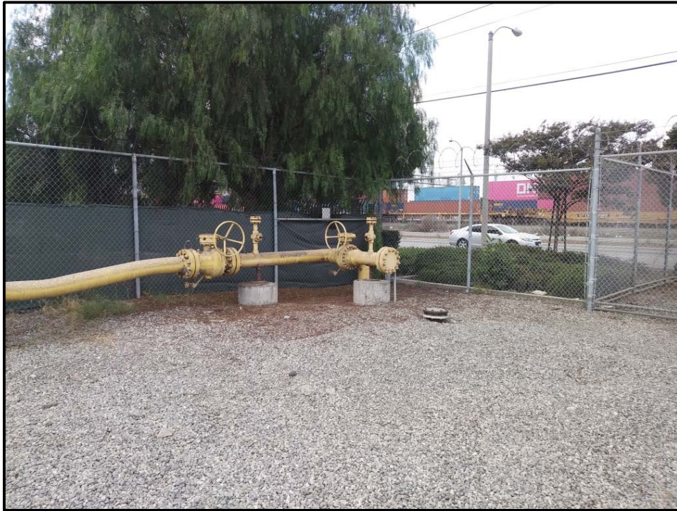
Figure 5-1. Western end of proposed pipeline, adjacent to South Alameda Street, facing west.
